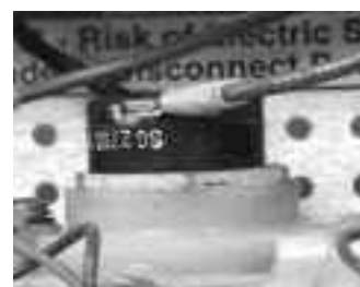
Figure 11: Installed heating element
